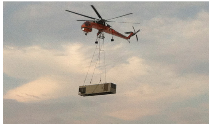
The helicopter positions a 90-ton Daikin RoofPak unit for the expansion facility—17 units set within 90 minutes
