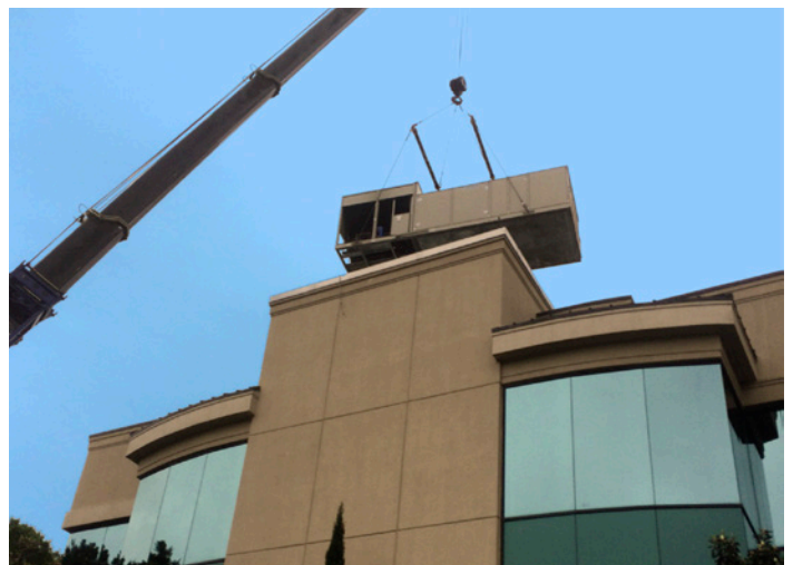
Installation of Daikin RoofPak units was staged over two weekends to ensure a successful retrofit.
