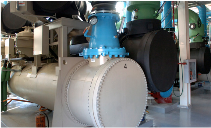
Regina General Hospital's two Daikin 1,350-ton dual compressor centrifugal chillers arranged in series counterflow.
