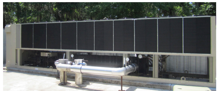
The 280-ton Pathfinder chiller with variable frequency drive provided improved efficiency and reliability.
