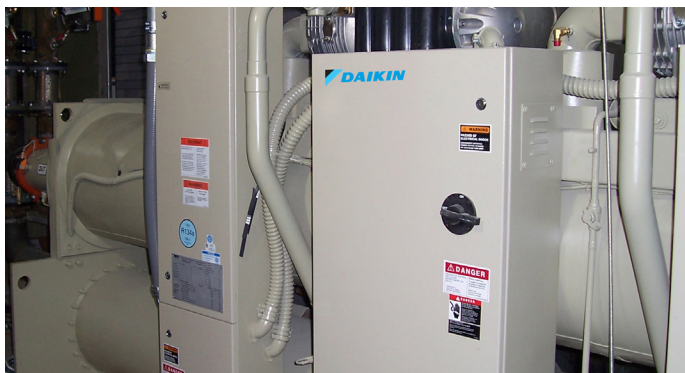
The chiller is immediately adjacent to a training space, but standing in that room, it's impossible to detect whether the chiller is on or off from a sound perspective.
