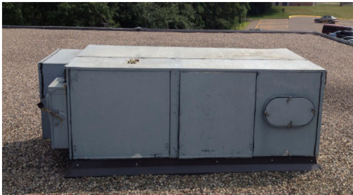
The resident halls' existing rooftop systems did not maintain adequate comfort levels. Rebel replacement units delivered improved comfort and energy efficiency solutions.
