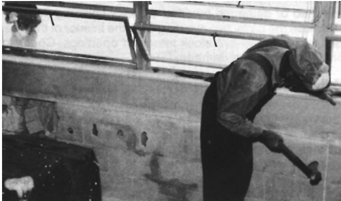
Figure 14: The interior wall is knocked out in the area cut for the wall sleeve
