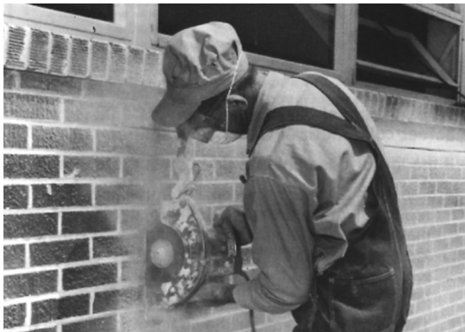
Figure 11: Cutting the outside wall rough opening slightly larger than the size of the louver
