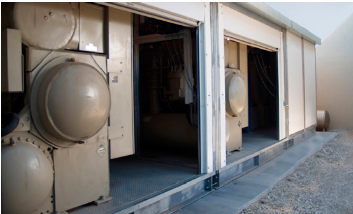
The Modular Central Plant at Chaparral High School features two energy efficient, 475-ton Daikin centrifugal chillers.
