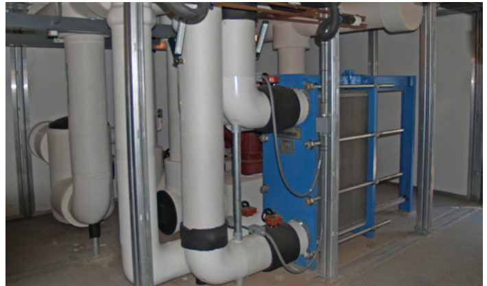
The Modular Central Plant at the school includes a plate-and-frame heat exchanger with secondary pumping.
