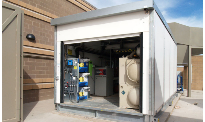
The Daikin Magnitude chiller, shown inside the MCP, contributed significantly to the energy savings for the Queen Creek Library.
