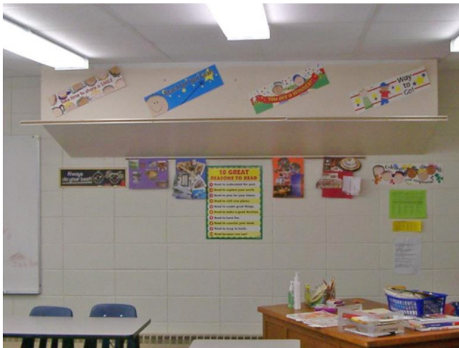
Figure 11: Room 33 – New HUV Now Above Ceiling Existing Outdoor Air Attenuator Remained in Place
