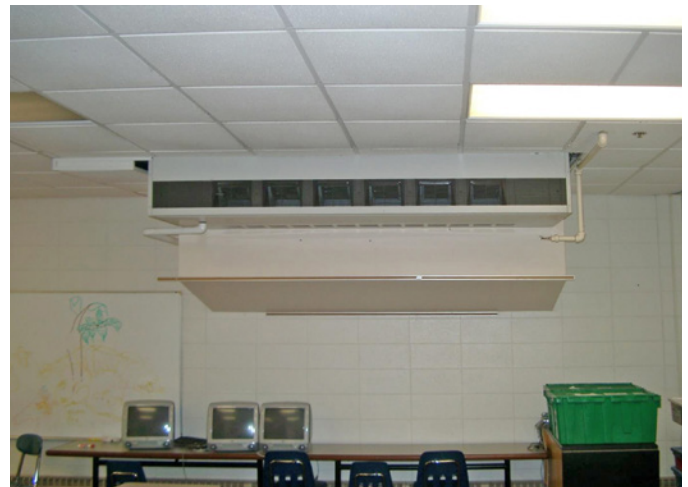
Figure 4: Existing Classroom 33 – HUV AAF Model AH-006
