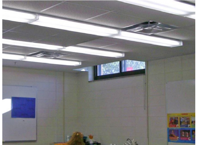
Figure 13: Room 35 – New HUV Now Above Ceiling, Existing Outdoor Air Attenuator Remained in Place
