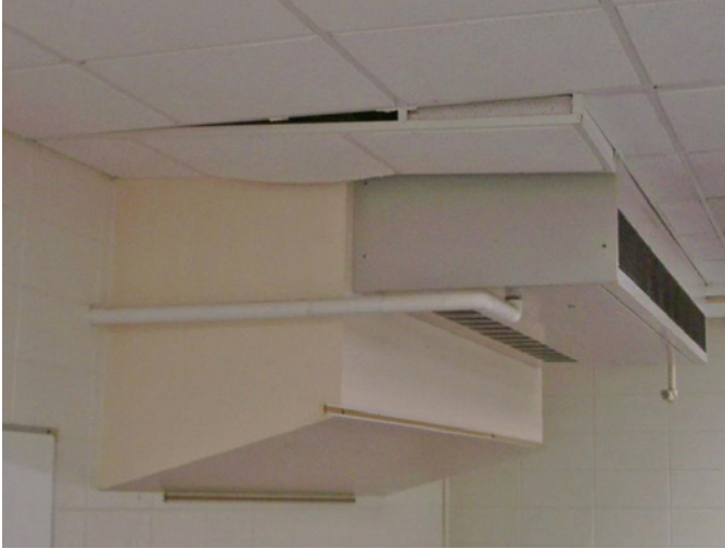
Figure 5: Existing Classroom 33 – HUV AAF Model AH-006
